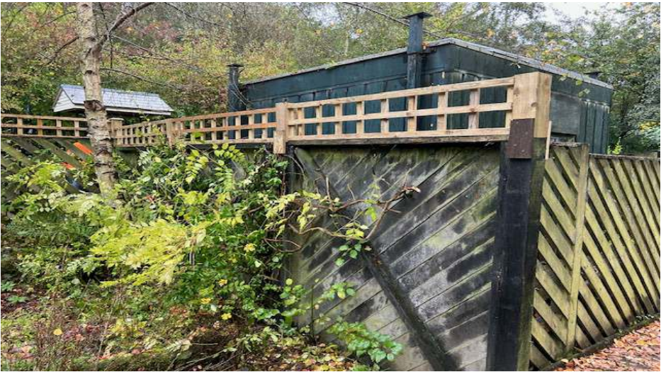
Part of the 20ft of new trellis during erection by the Friends in the Chelsea Gardens
